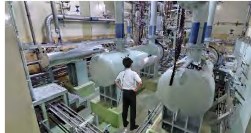
Confirmation of work site (The data is from Fugen) (Realistic sense of presence, checked with worker's eyes)
