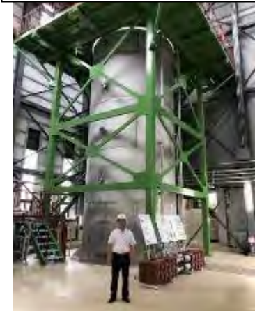
Cylindrical Water Tank
